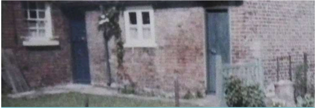
Typical single storey scullery showing the back door (left) and the door to the outside toilet
